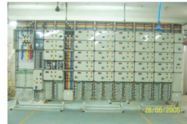
MCC Panel Installed at JK Paper Ltd
