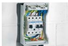
British Standard installation with earthed armoured cables
