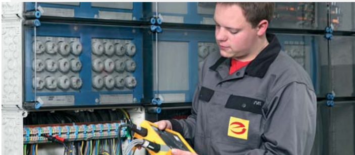
Power distribution board (PSC) in accordance with IEC 61439-2
