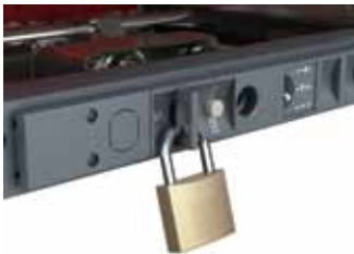
“Disconnected” position locking by padlock.
