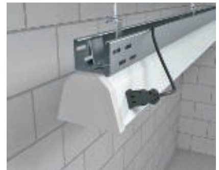
Pre-wired luminaire supports Mounting of a pre-terminated luminaire beneath a luminaire support tray.
