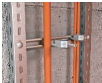
Cable fastening with U clamp Fastening of a cable to the rung with U clamp.
