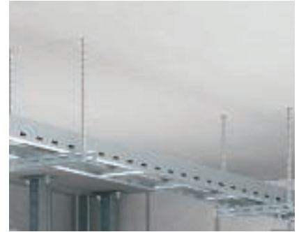
Threaded rod suspension application Suspension of a cable ladder with threaded rods and U supports as a cross-section.
