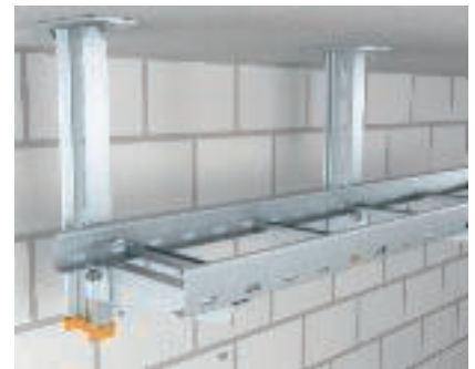
Support suspension Suspension of a cable ladder with supports and support brackets.
