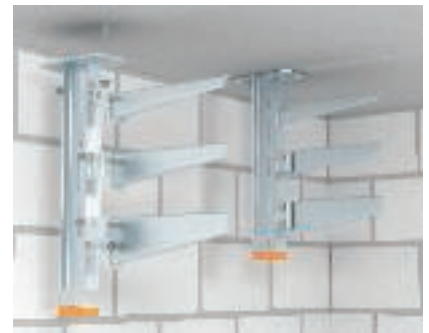
Bracket mounting Installation of a three-layer cable support system on the concrete ceiling using support bracket mounting, AS 15, AS 30 and AS 55.
