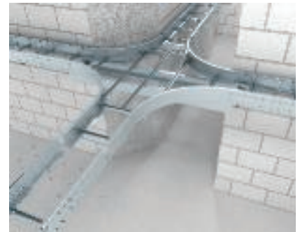
Installation of cross-over Cross-over in combination with wide span cable ladder. The cross-over is connected to the wide span cable ladder using external connectors.
