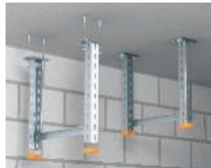
Traverse Installation of U supports US 3 K, US 5 K and US 7 K under the ceiling using anchor bolts, FAZ II, and use of a trapeze, consisting of U profile US 3, US 5 or US 7.
