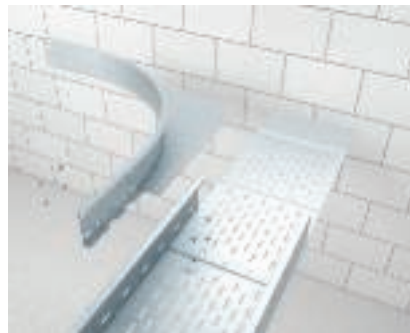
Creation of a tee with add-on corner Installation of the first add-on corner, type WEAS 110.
