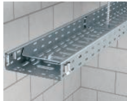
Installation of central suspension MAH 60 Insertion and alignment of the central suspension, MAH 60, in the cable tray.
