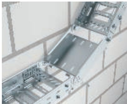
Installation of adjustable vertical bend element Installation of the adjustable vertical bend element for the creation of adjustable bends. The adjustable vertical bend element is connected to the cable tray using adjustable connectors.
