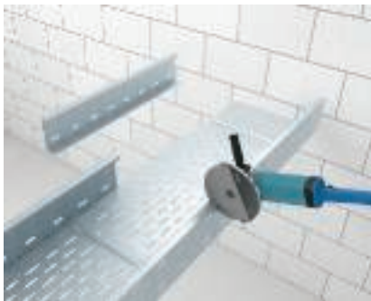
Creation of a tee with add-on corner Removal of the side rails from the wide span tray.
