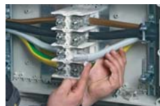
Conductor ends need to be rubbed with an acid and alkali free grease and immediately connected
