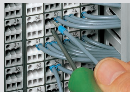
Connection of ferruled wires
