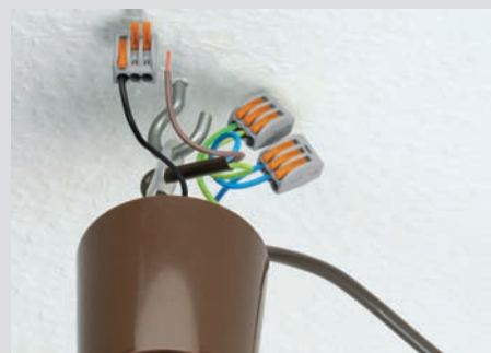
Lighting fixture connection with flexible conductors and power feed
