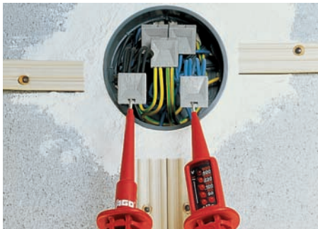
Voltage testing at push-wire connectors
